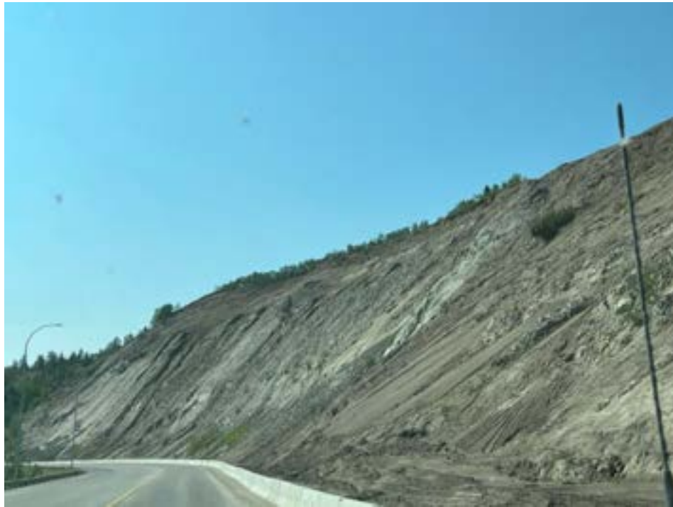
Photograph 3. High erosion constraint. Steep slope with visible sloughing.
