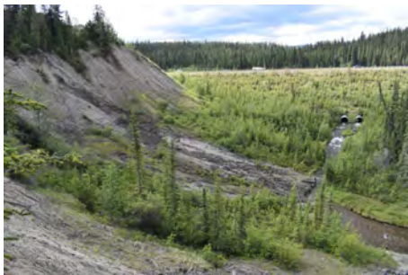
Slope failure by McIntyre Creek
