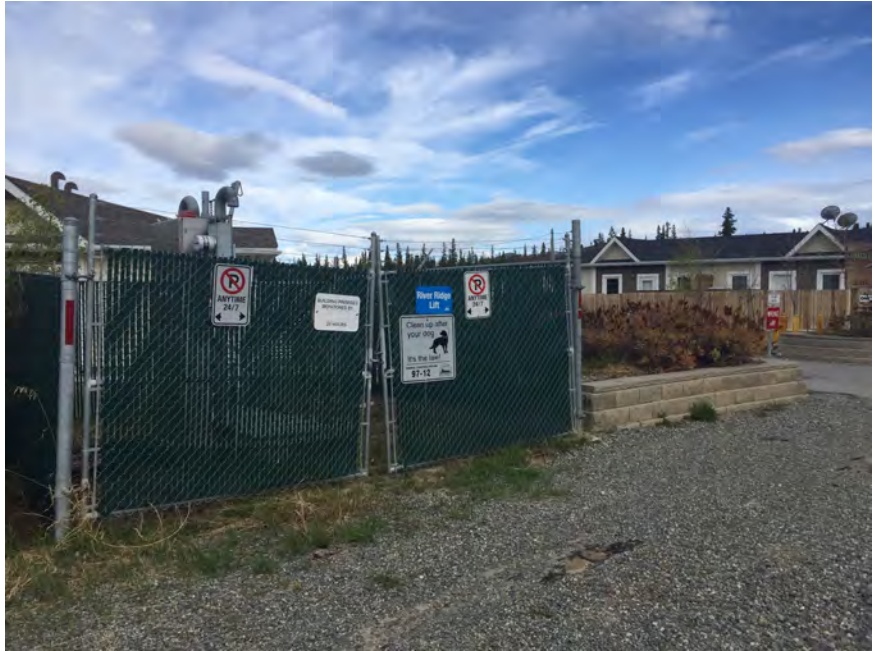
River Ridge lift station
