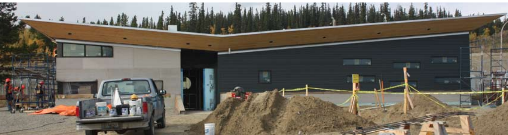
BELOW: The Transitional Women's Living Unit at the jail is being built by KDFN crews.
