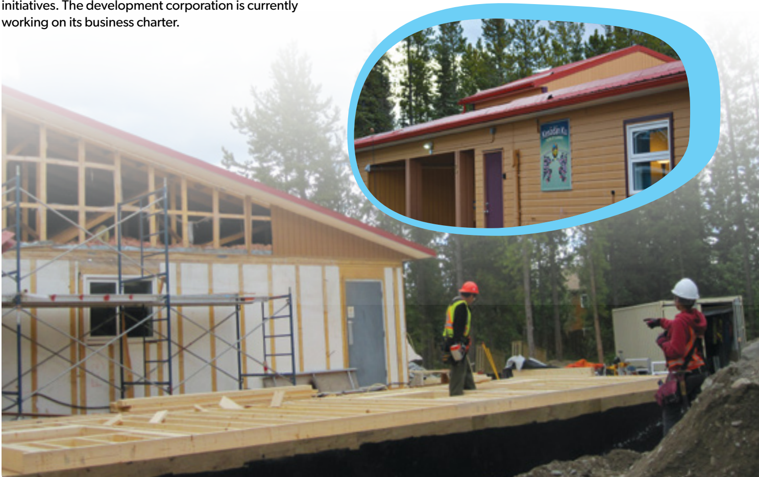
Work in progress during the House of Learning expansion (inset of completed building). Funds for the project were provided through a Yukon Asset Construction Agreement connected to the FH Collins construction project.
