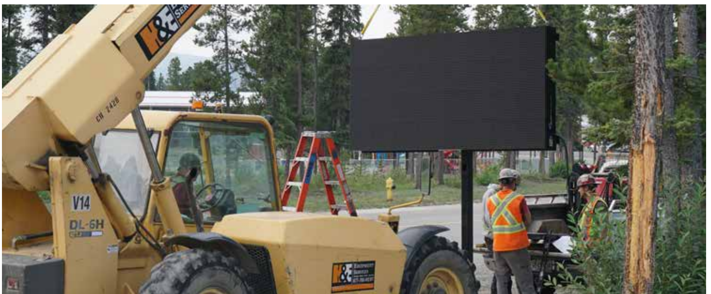
The digital sign being installed in front of the Nàkwat'á Kù Potlatch House this summer.
